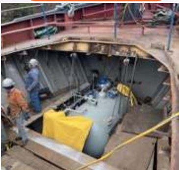
NH 3 tank & feed
